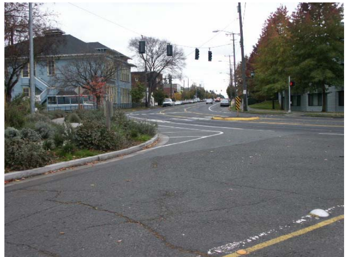
Tight Curb Radii, Seattle WA
