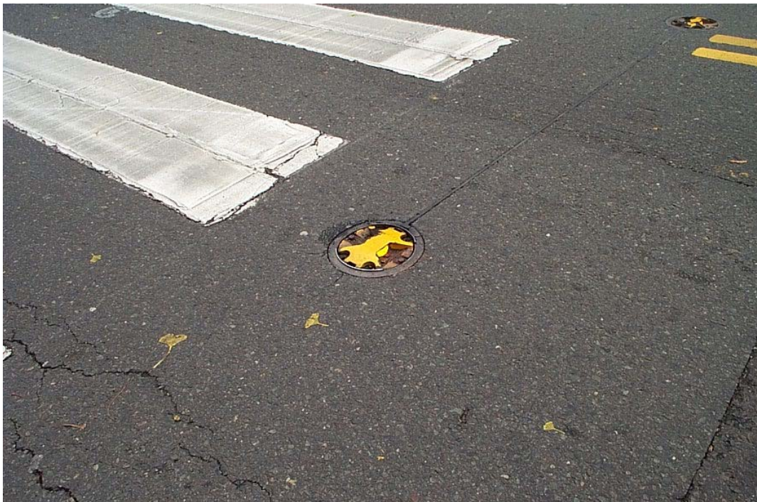
In-Pavement Flashing Pedestrian Warning Lights, Cambridge MA
